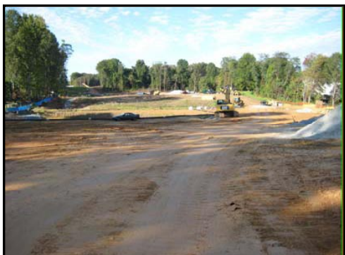
A view of the ICC in Contract A looking west from Shady Grove Road towards I-370.
