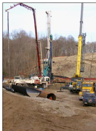
Pumping concrete for caissons at the bridge over North Branch Rock Creek in Contract A.
