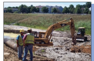
Demucking a pond and converting it to the permanent stormwater management facility.
