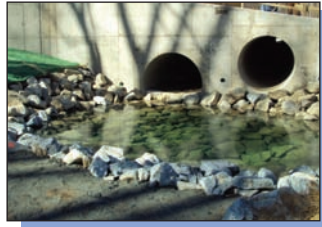
This culvert is designed for small mammal and amphibian passage.
