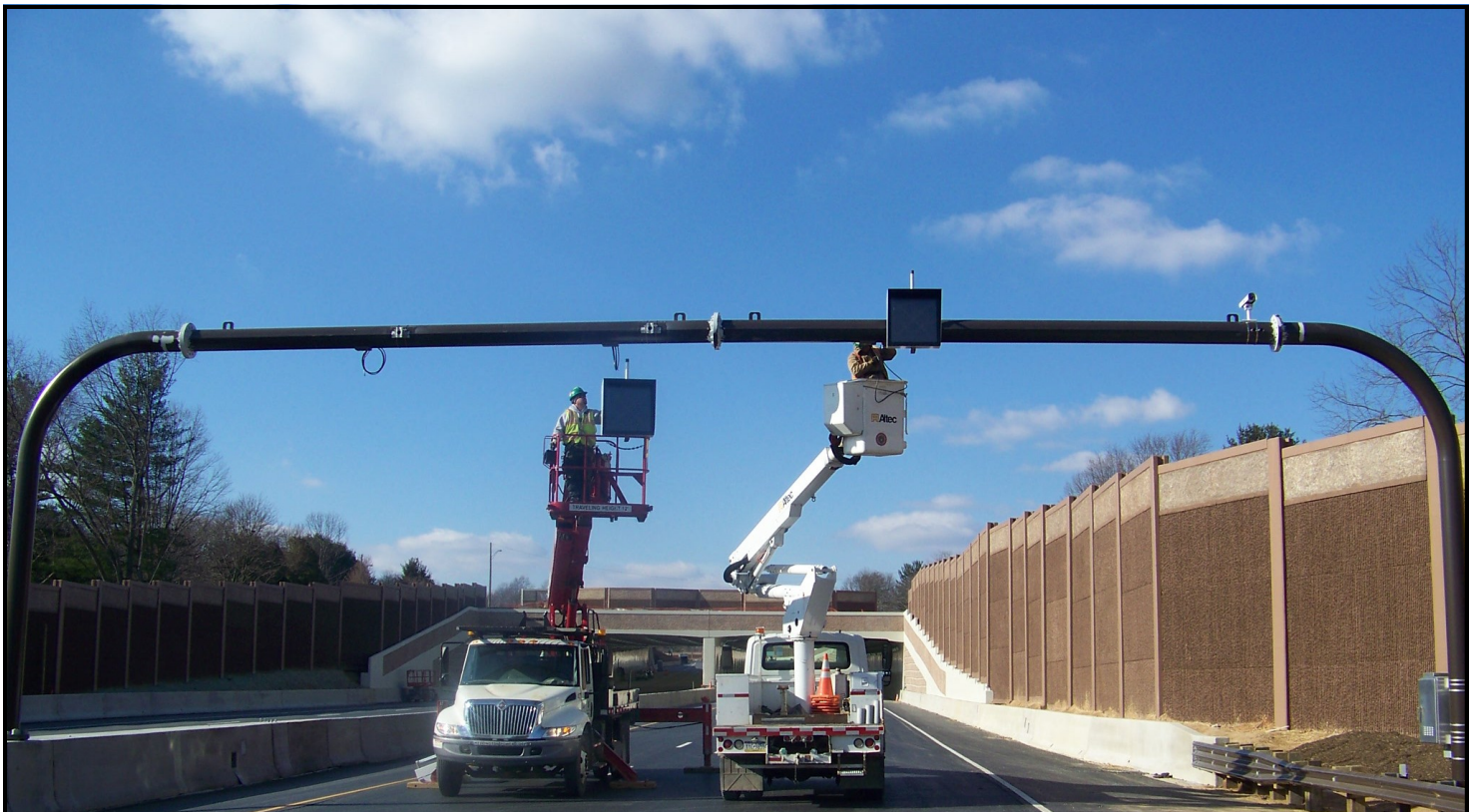
Installation of lane-use control signals near Olde Mill Run Deckover
