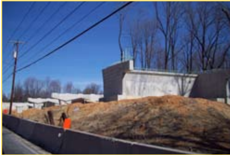
Construction is underway on the new bridge that will take Old Columbia Pike over the Intercounty Connector.
