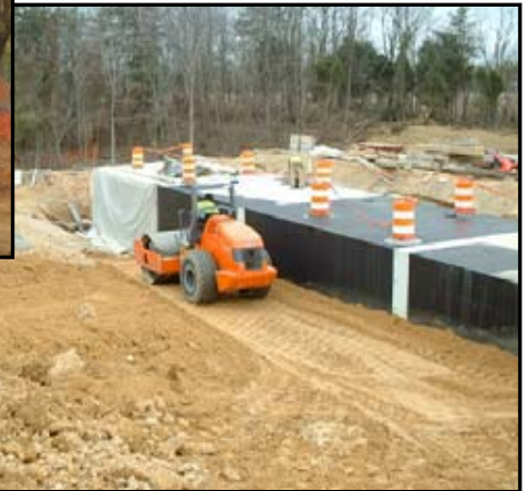
Contract C: (Above) Compacting backfill for a box culvert east of Old Gunpowder Rd.
