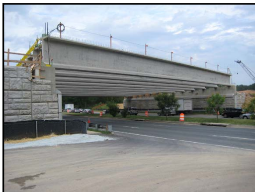
Photo 1- Contract A: Concrete girders for the ICC bridge over Shady Grove Rd.
