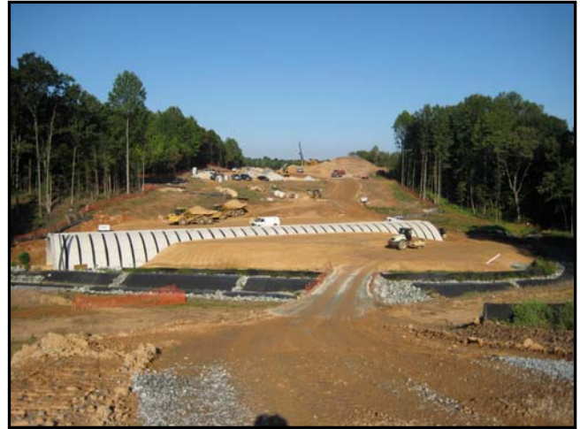
Contract A: (Above) Looking west from Redland Rd. past the bottomless culvert over a tributary to Mill Creek.
