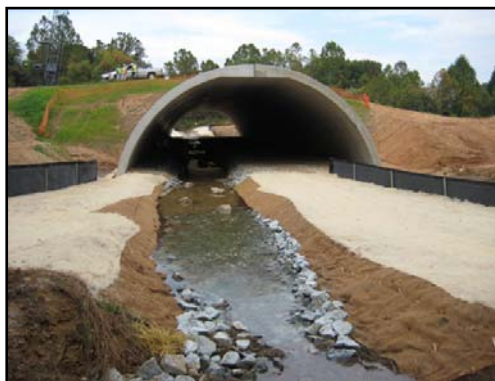
Designed as a passage for wildlife, Mill Creek runs through this BEBO culvert in Contract A.
